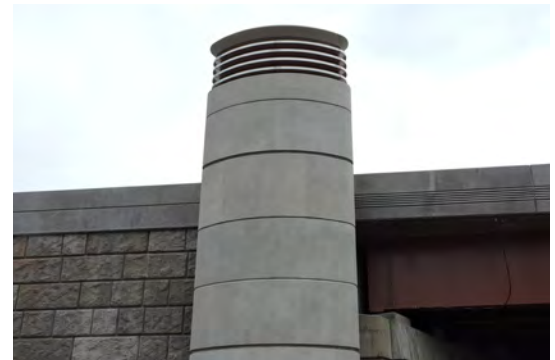
The completed bridge carrying I-95 over Canal Dock Road was designed to provide a distinctive gateway to New Haven's waterfront
